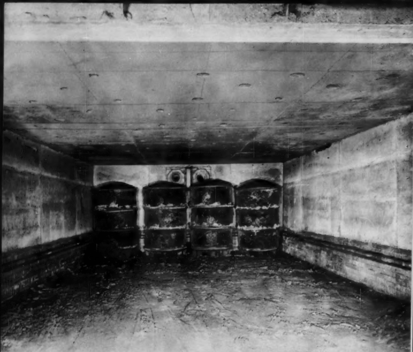
SIDE WALLS AND FLAT ARCH ROOF on this batch-type annealing oven at Terre Haute Malleable & Mfg. Corporation, Terre Haute, Indiana, were installed quickly and economically with a castable refractory—Kast-O-Lite—a Lumnite-base castable manufactured by A. P. Green Fire Brick Company, Mexico, Mo.
